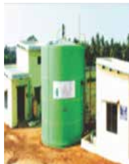
Distributed Biogas Plant
