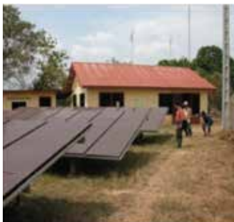
Distributed Solar Plant
