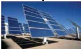
Solar Power Plant
