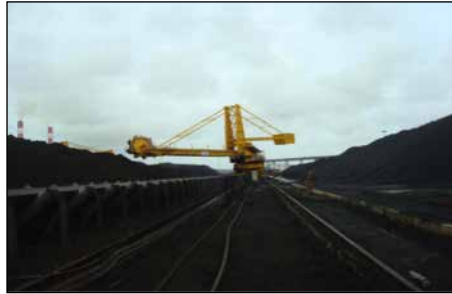
Pic 2.4: Stacking system
