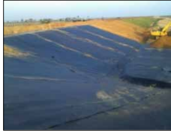
Pic 8.8: Ash pond liner
