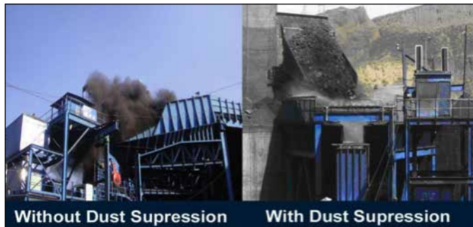
Pic 2.11: Unloading station dust suppression
