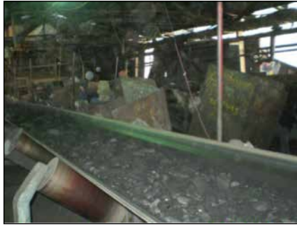
Pic 3.1: Enclosed coal conveyors
